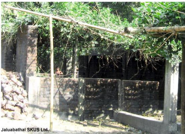
The present condition of the godown at Jaluabathal (sanctioned in 1995-1996) as of February 2008
